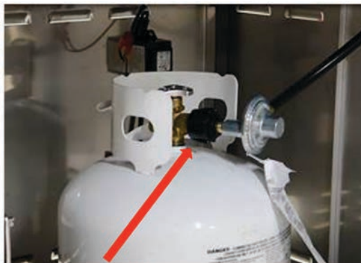
Regulator connected to propane tank.
